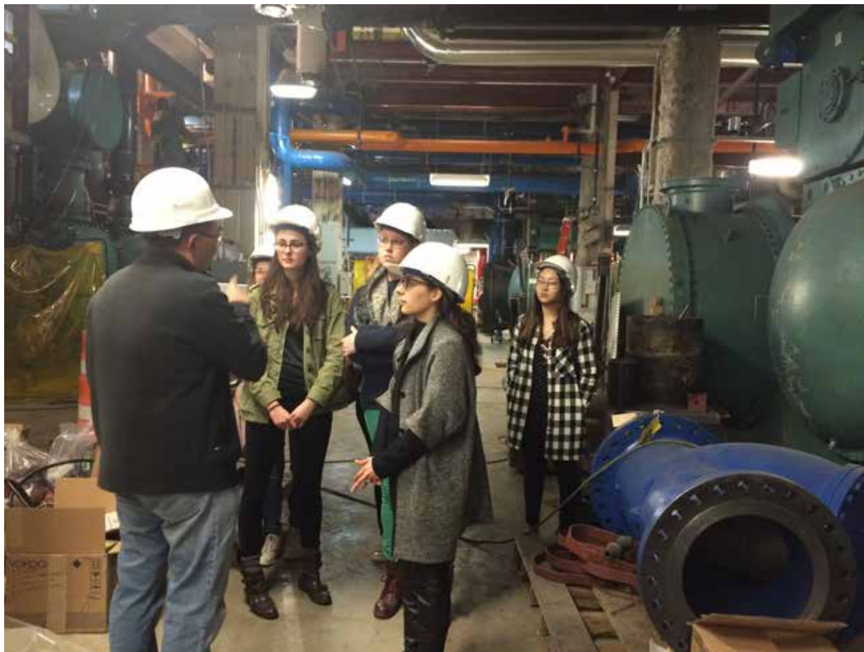
The Sloan-supported Women in Energy program at Columbia's Center on Global Energy Policy seeks to help grow the presence and leadership of women in the energy sector. Here, program participants visit Columbia University's Central Chiller and Boiler Plants. (PHOTO COURTESY OF COLUMBIA CENTER ON GLOBAL ENERGY POLICY)
